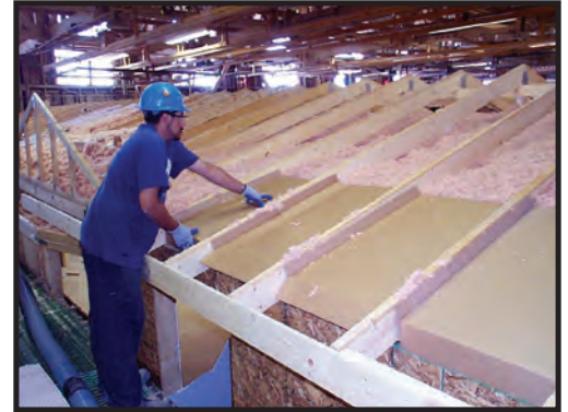
Building in a climate controlled environment reduces costs by protecting materials from the elements
